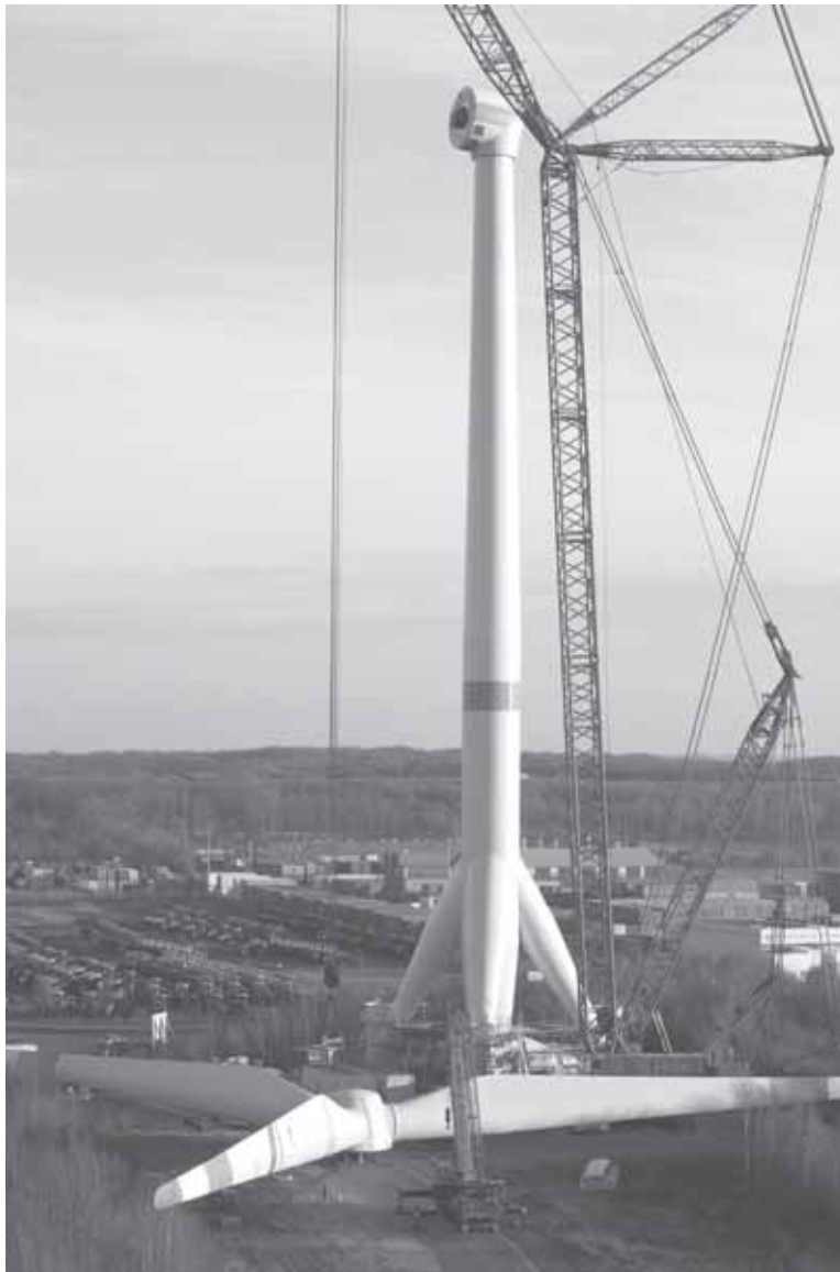
Figure 6 M5000 construction on shore in Bremerhaven at an offshore tripod foundation. Source: Multibrid Entwicklungsgesellschaft Ltd.
